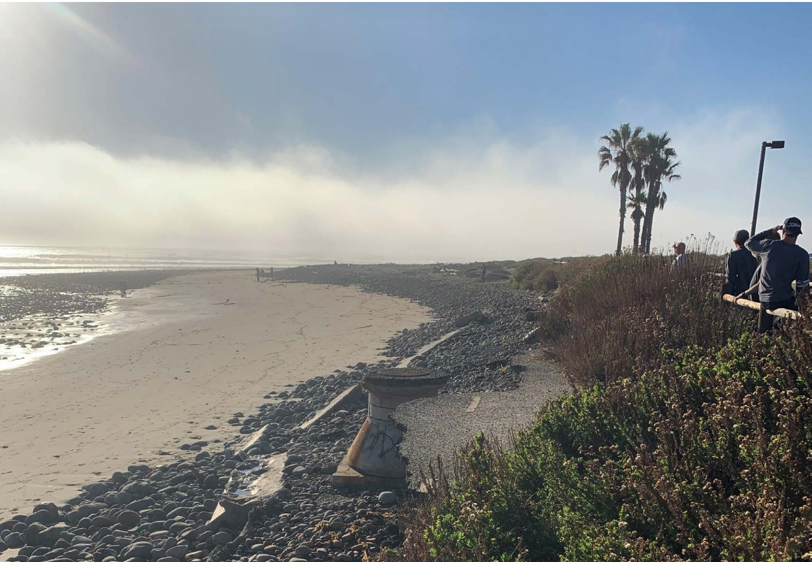
Surfer’s Point Managed Retreat Project, City of Ventura. Damaged bike trail due to erosion.
