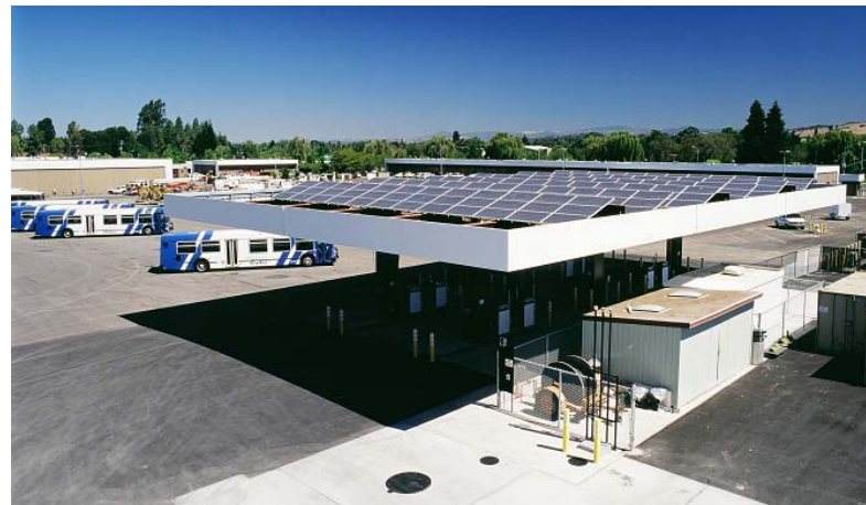
Fueling Station: 29.3 kW
