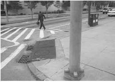
A curb cut located outside Atlanta's City Hall. The location of the sewer grate makes it almost impossible for a mobility impaired individual to cross the street.
